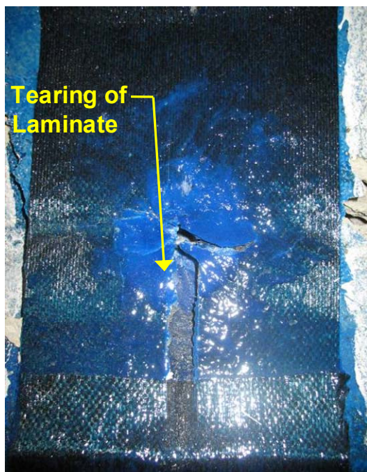
Figure 7.35 – B-4a Failed Laminate
