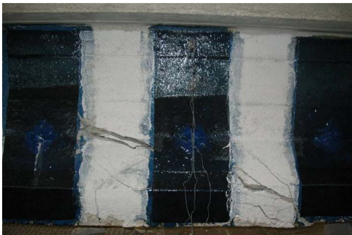
Figure 7.34 – B-4a Failed Section
